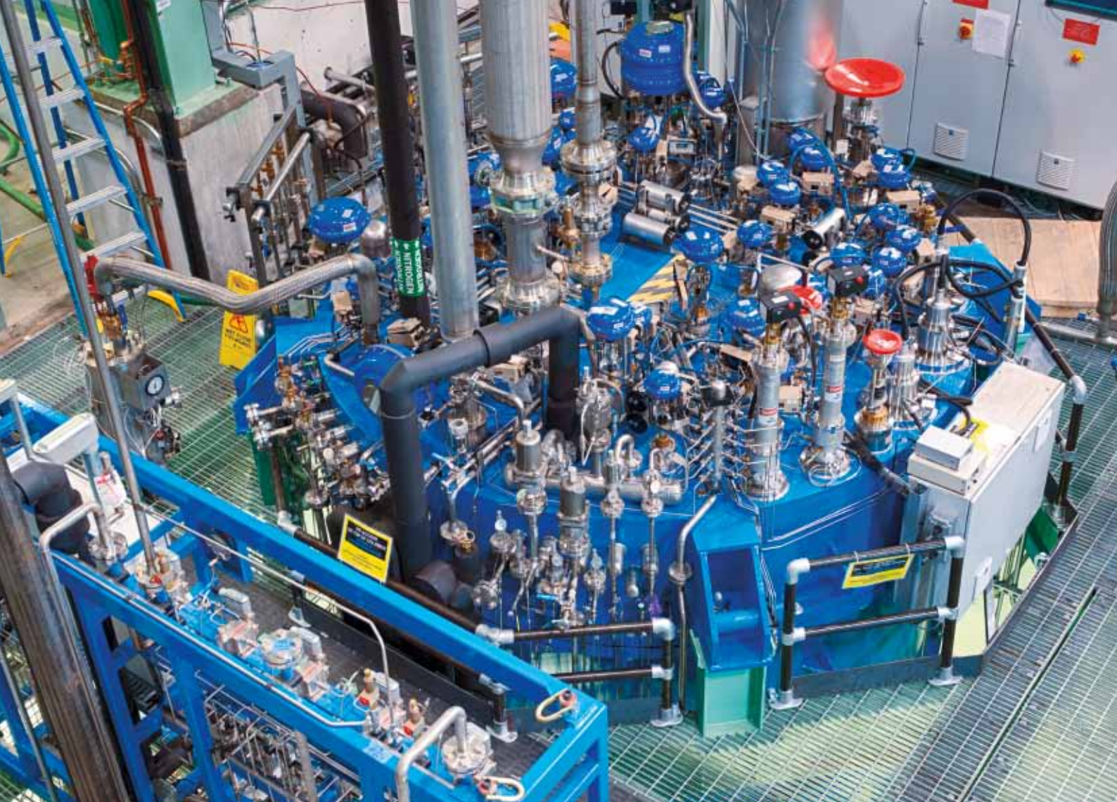
The interior complexity of the superfluid helium refrigerator coldbox can be seen from the tight arrangement of components on the valve plate (above). Picture: © Fermilab
