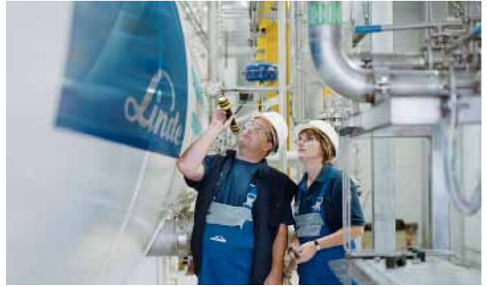
Hydrogen liquefaction plant in Leuna, Germany.
